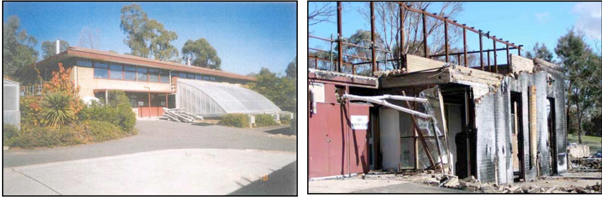
Figure 1: The main building (left) before and (right) after the fire. The stores were located at the far end of the building as show in these pictures. (Photo on left from Egan Insurance Report)
